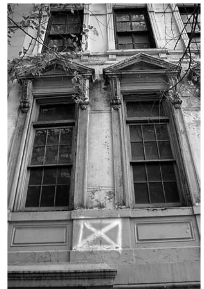
An ominous yellow x covers the deteriorating façade of 114 East 76th Street
